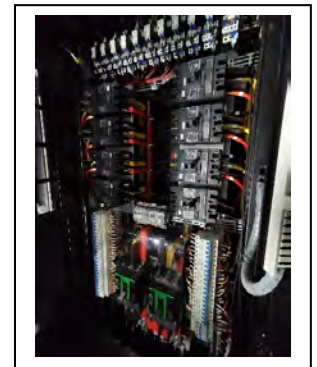
Power Cabinet Box
