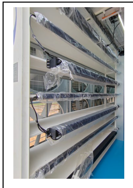
PDU on the Racks
